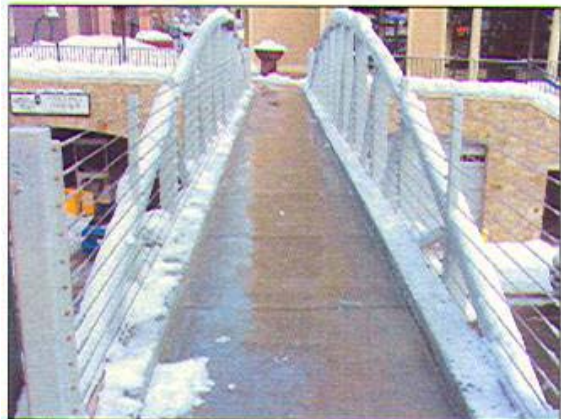
The Tuff Cable, a copper cable, is used in snowmelt systems for driveways or sidewalks. In an existing driveway, technicians cut thin, inch-deep channels that are 6 inches apart into the pavement, which is where the cable is laid and then closed with a sealant.
